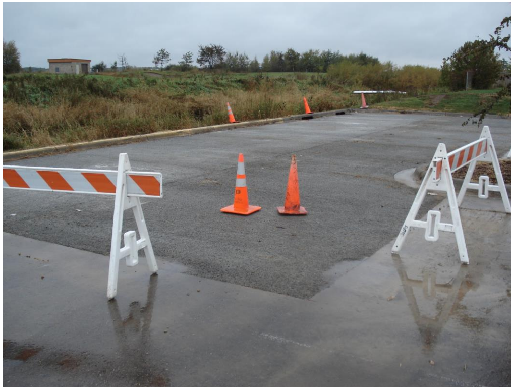
Pervious Concrete, National Sports Center Super Rink, October 2009
