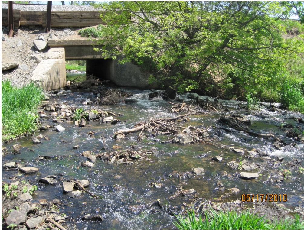
BNRR Riprap Obstruction May 2010
