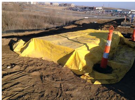
Cover materials using tarps or plastic sheeting to prevent precipitation from contacting construction site materials. Direct work crews to replace material stockpile covers at the end of the day and before rain. Photo credit: Barry Tønning, Tetra Tech
